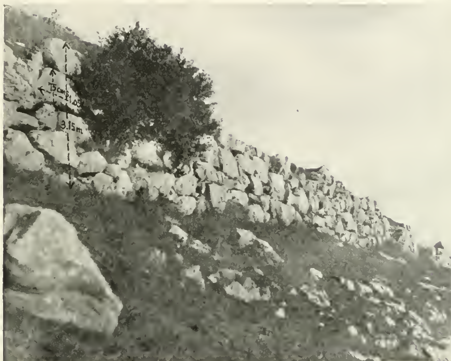
FIGURE 4. — A PIECE OF THE OUTER WALL ON THE WEST SIDE Near point A, between the posterns at Nos. 6 and 7
